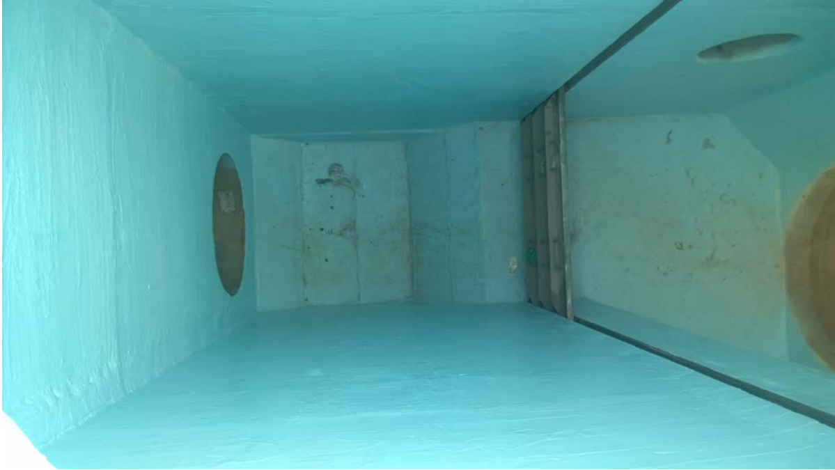
Figure 3. Top view of eastern 36-inch inlet pipe of the Downstream Siphon Structure inlet pipes showing stop logs installed. Also shown is the 60-inch outlet pipe and the 18-inch inlet pipe.
